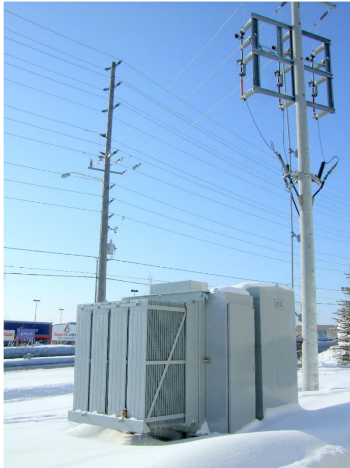
Figure 2: Pole Mounted Switch and Transformer
